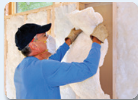
Proper insulation holds heat inside during the winter and keeps it from coming in during the summer.
